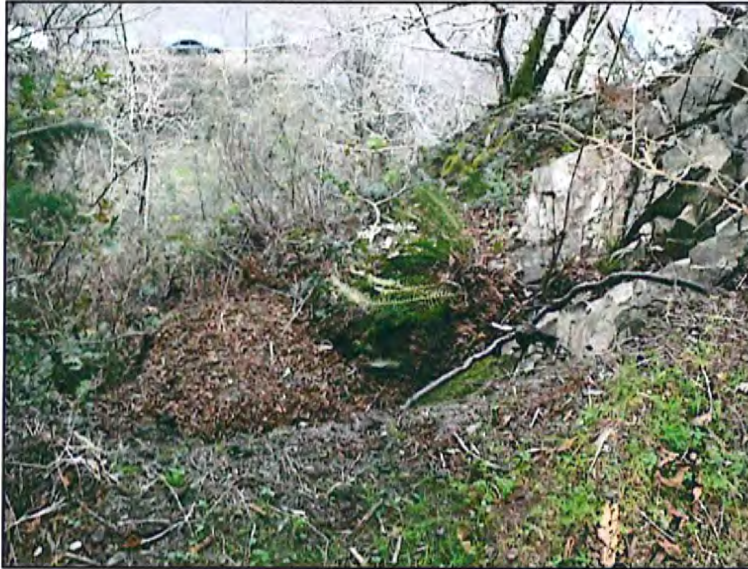
East of 1600 Coxcomb Hill Rd Cliff Erosion
